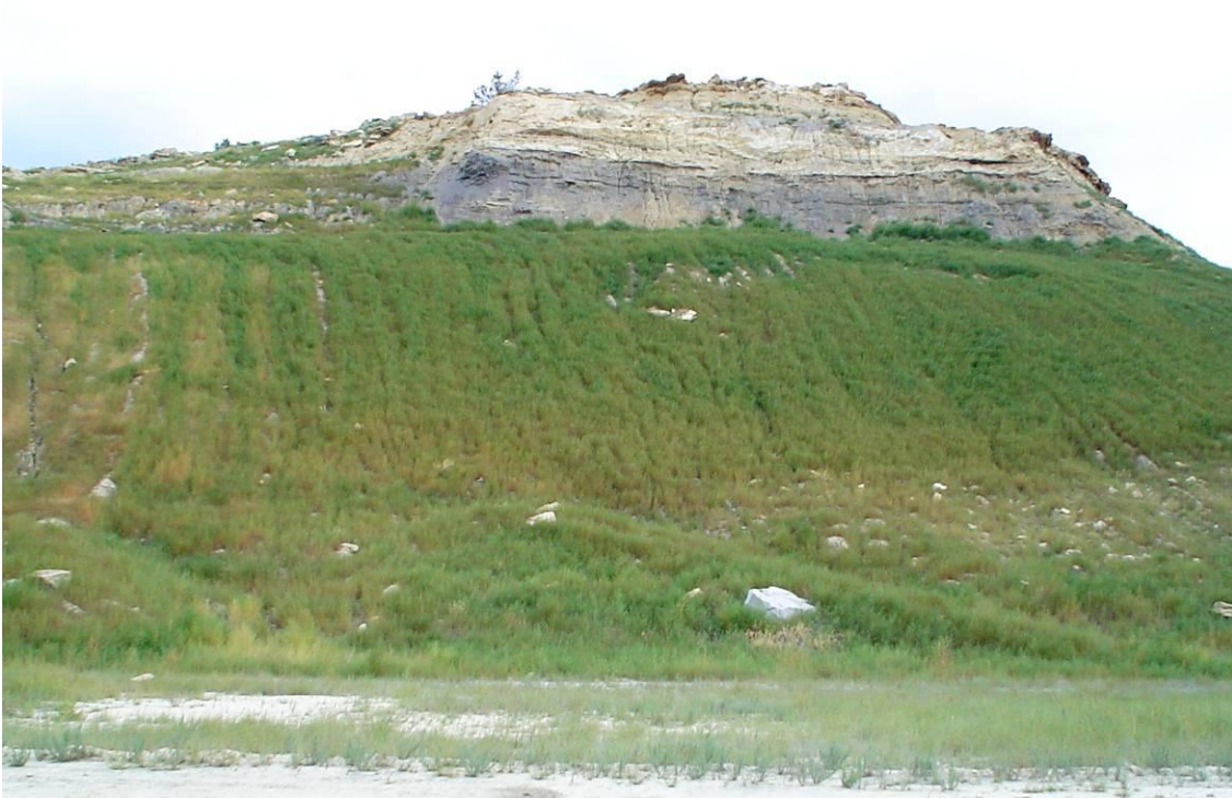
Figure 5. The rilling on this slope is the result of inadequate drainage density coupled with incorrect longitudinal profile.
